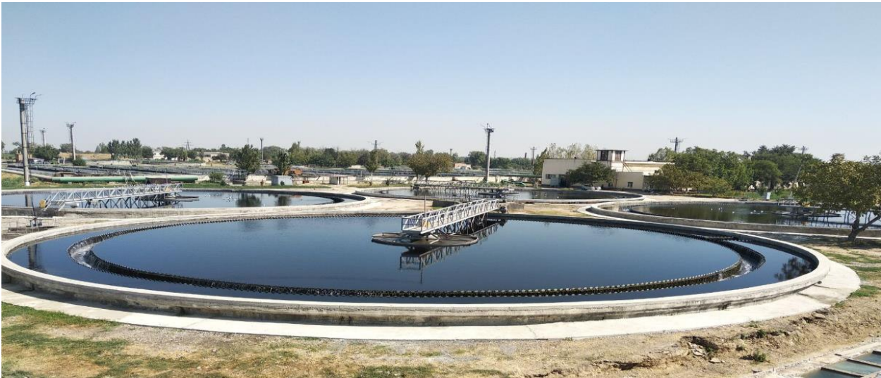
Figure 4. Bozsu aeration station
