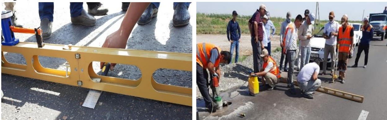
Figure 1: Measurements of wheel track defects on public highways using a 3-meter ruler
